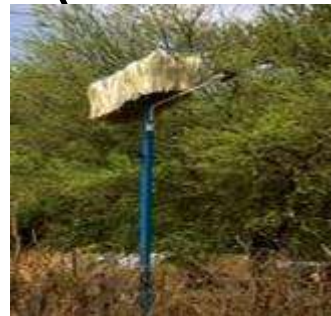
Solar street lighting
