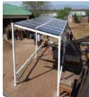
Solar energy for buildings
